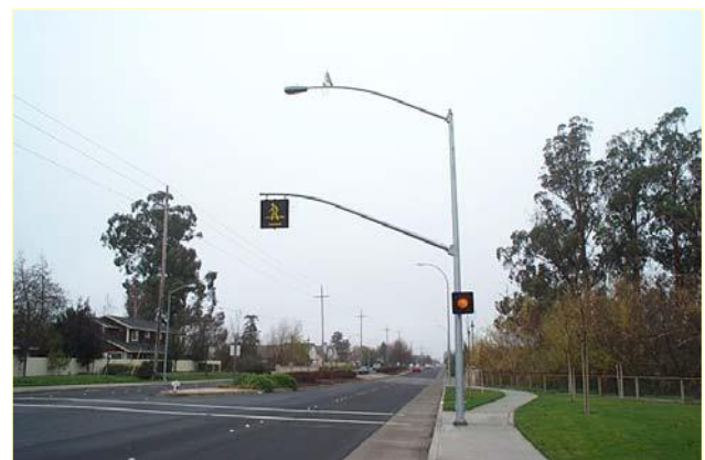
Overhead Pedestrian Warning and Flashing Beacon
